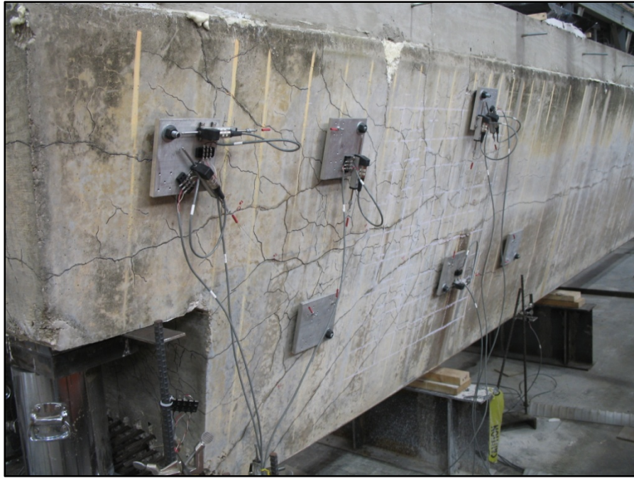
Figure 3-22 Crack measuring/shear distortion instrumentation installed at reentrant corner and in web.
